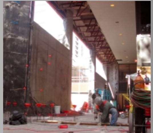
The new hydrostatic wall between the JFB building and the Medical School takes shape.
